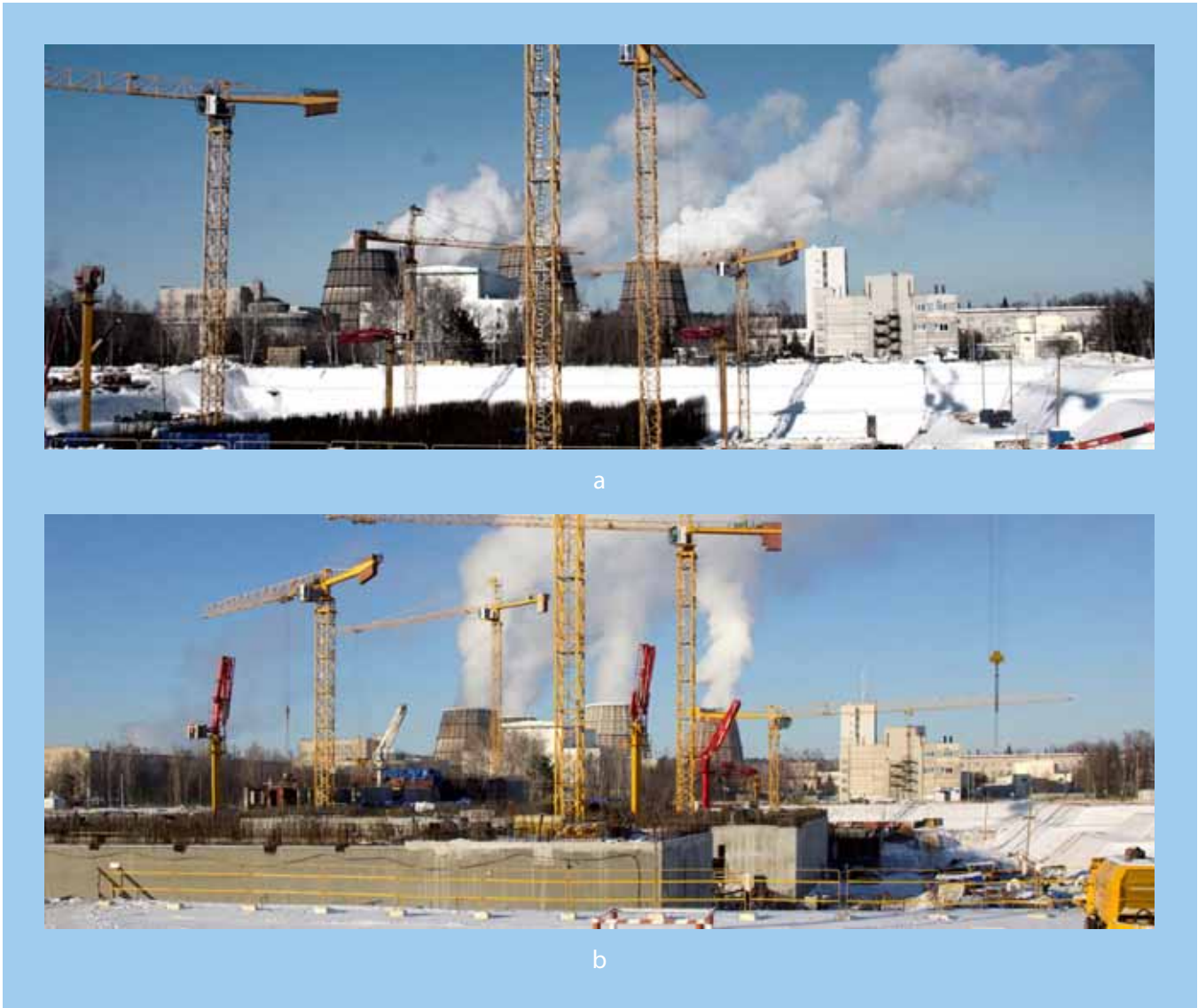
Fig. 4.2.7. Overall view of the MBIR area at the beginning of (a) and by the end (b) of 2016
