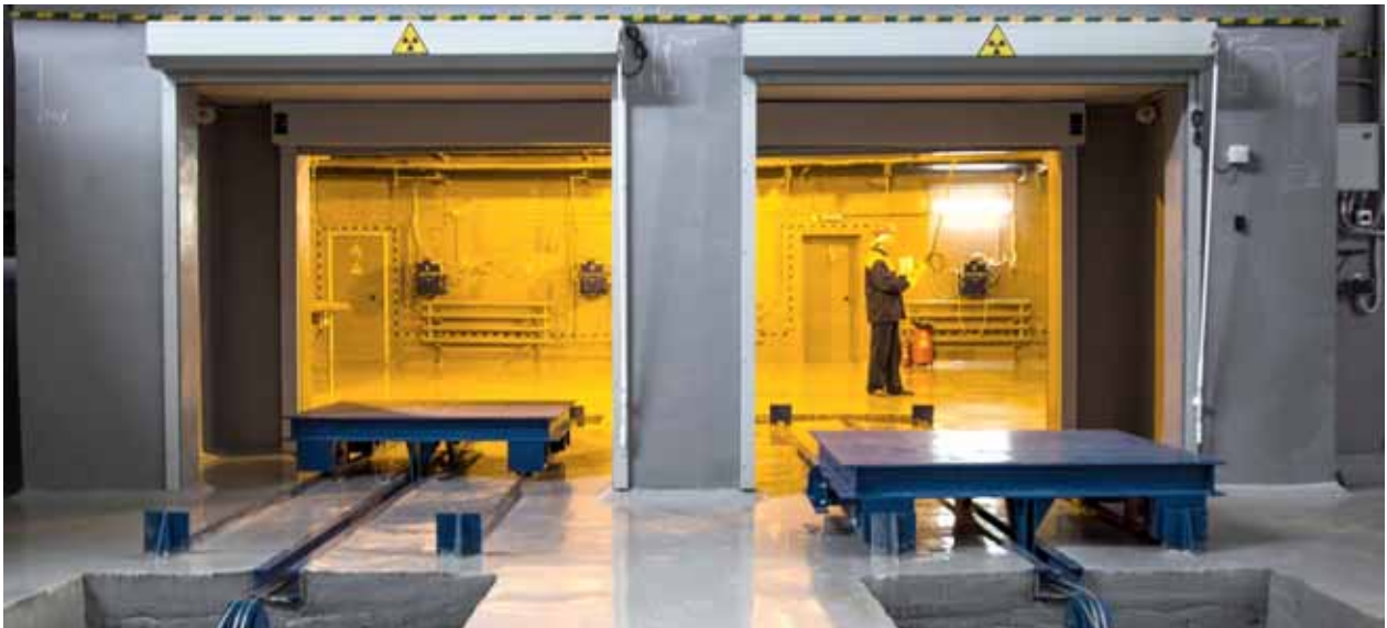
Fig. 3.6.8. Solid radioactive waste storage facility
